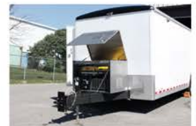
External Generator Cabinet
