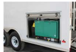
Internal Generator Cabinet
